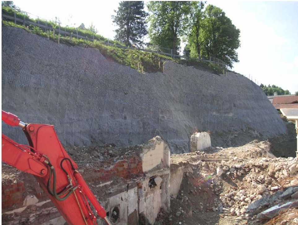
Fig. 7: Beginning the excavation work for the foundation of the apartment houses, with adjoining finished stabilised steep slope
