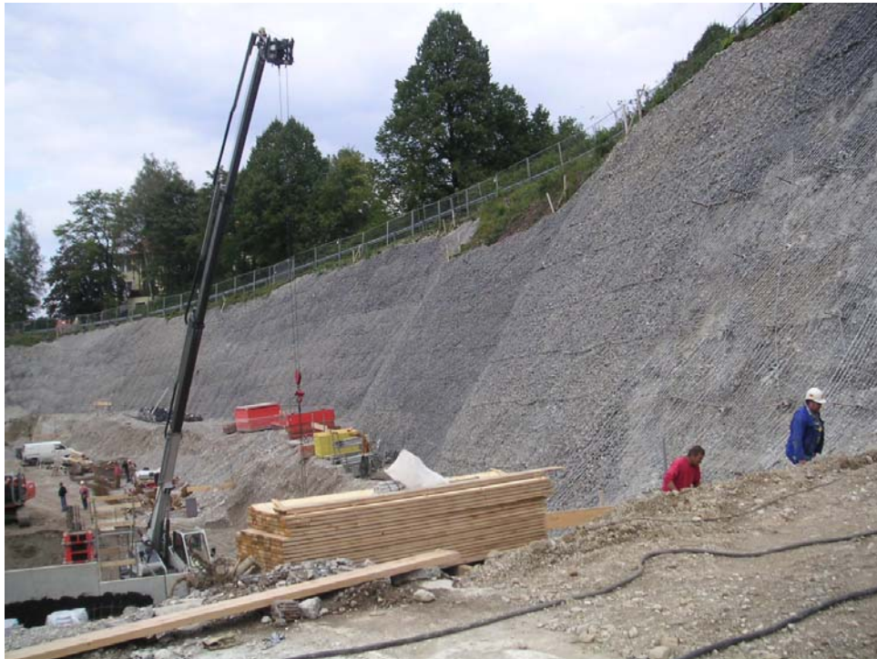
Fig. 9/10: Filling of the anchored lattice mats with gravel, grain size 32/60 mm, Volume approx. 7 - 8 m 3 per 100 m 2
