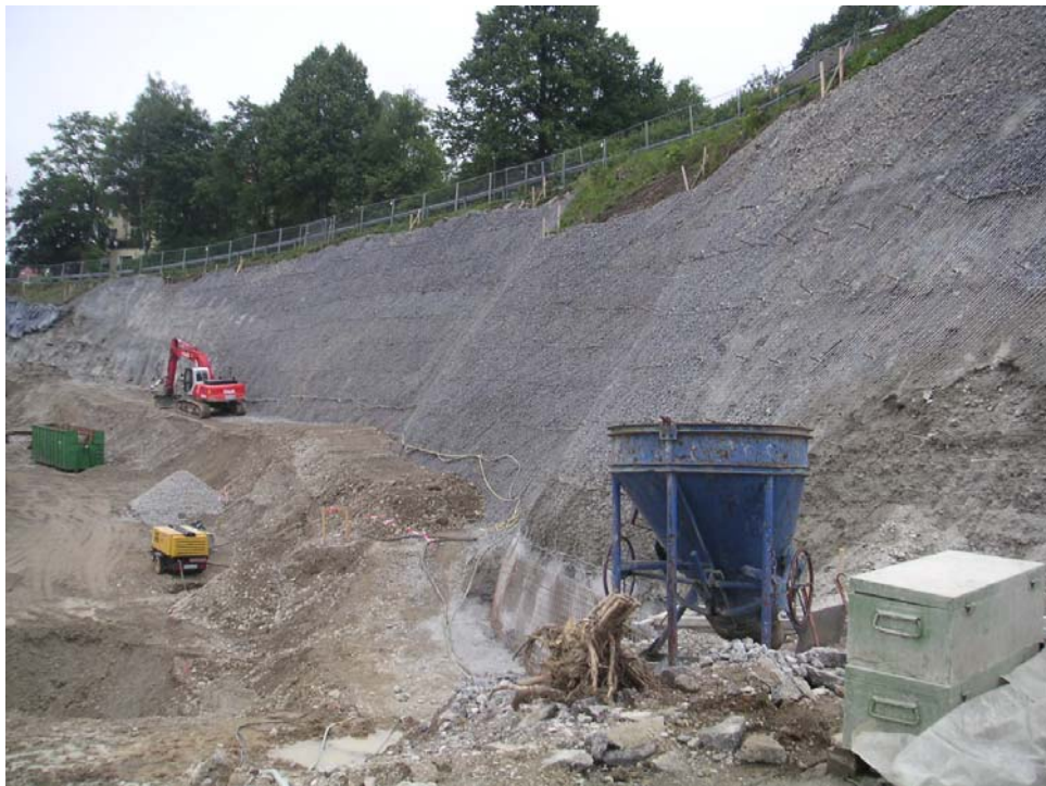
Fig. 8: A crane bucket (in the foreground) with an opening on the side for stone filling
