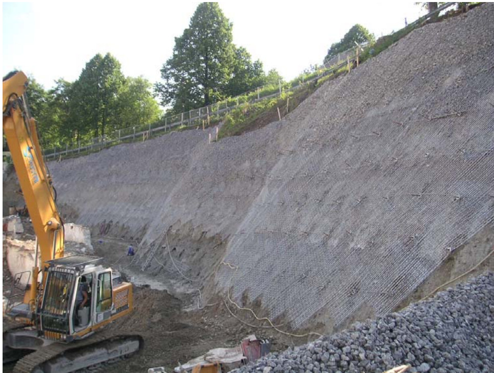
Fig. 6: Finished cut slope, inclination 65°, down to the level of the floor of the excavation pit for the foundation
